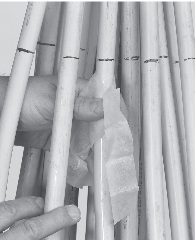
2.2 Clean and abrade the MDF cables over a distance of 150 mm from the mark downwards.
